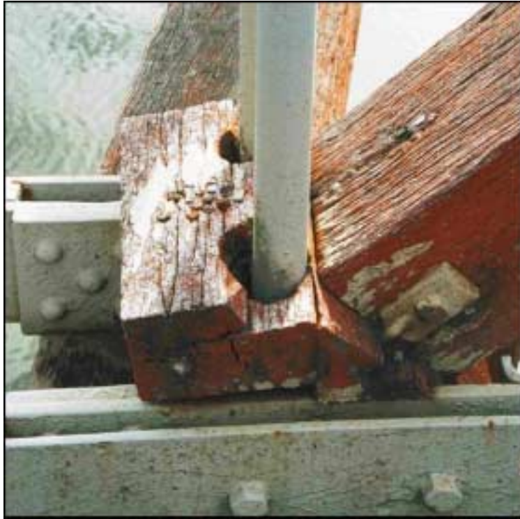
Figure 5: Deterioration of a Typical Thrust Block
