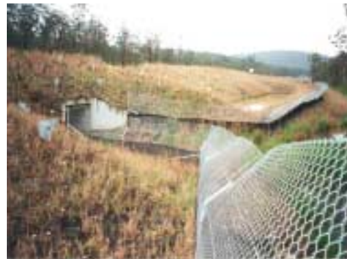
Fig. 18: Placement of fauna fencing (floppy top type) at a fauna underpass entrance.
