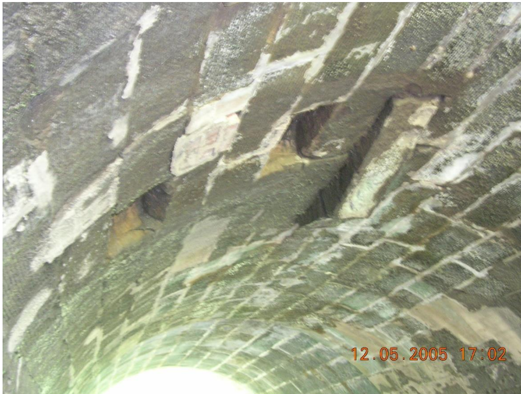
Figure 1 GSW bridge with broken voussoirs
