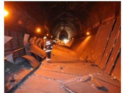
Progressive collapse (Sasago tunnel)
