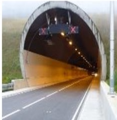
Tunnel ventilation and information systems
