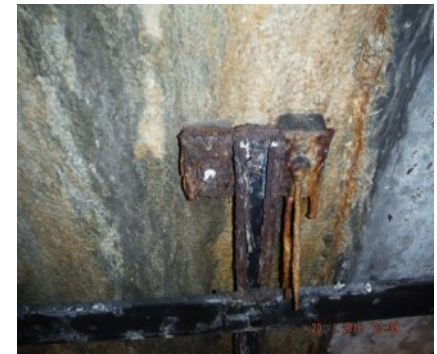
Corrosion of hidden fixings
